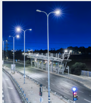
LED LIGHTING SMART LIGHT POLE
