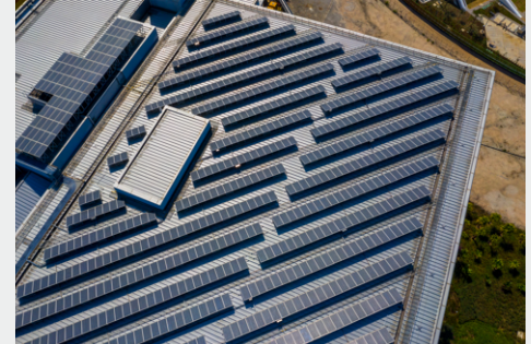
SOLAR / ENERGY STORAGE
