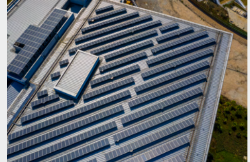
SOLAR / ENERGY STORAGE
