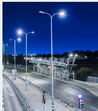
LED LIGHTING SMART LIGHT POLE
