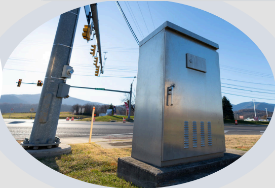
Traffic Signal Control
